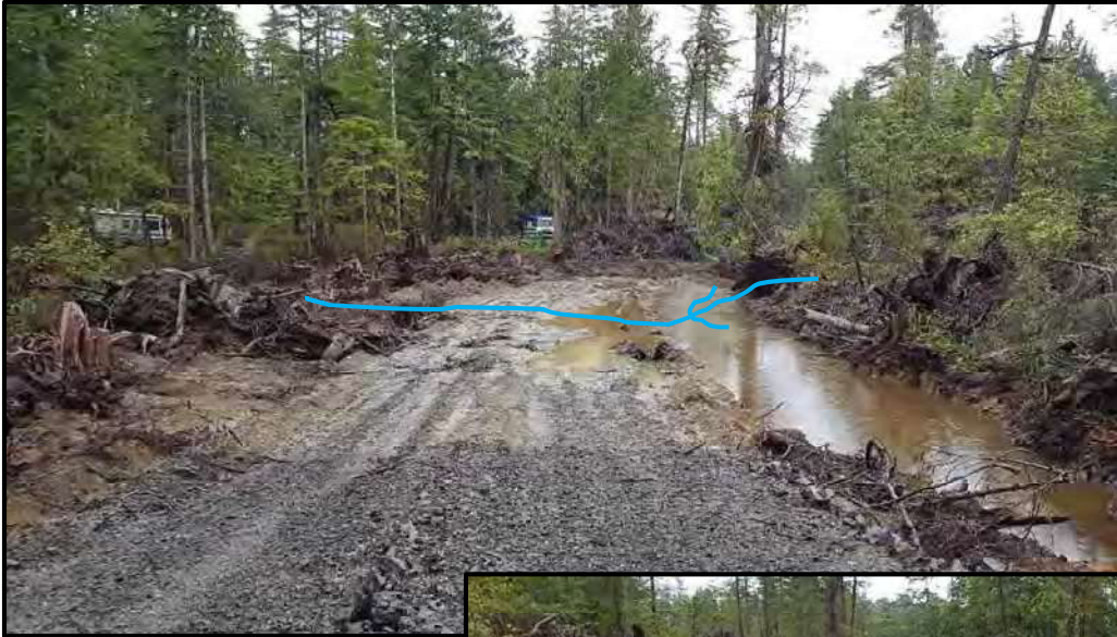
Photo 7: View on opposite side of road alignment. Pondered water along road at upper end of the Middle Stream side channel; Southern half of property.
