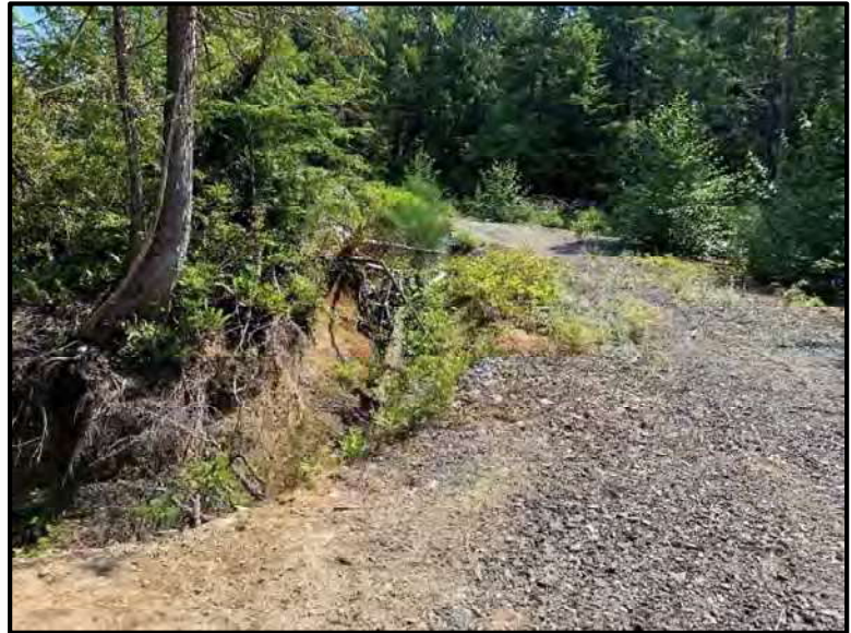
Photo 15. Gravel loop road through southern section of the site with deep ditches along the sides of the road.
