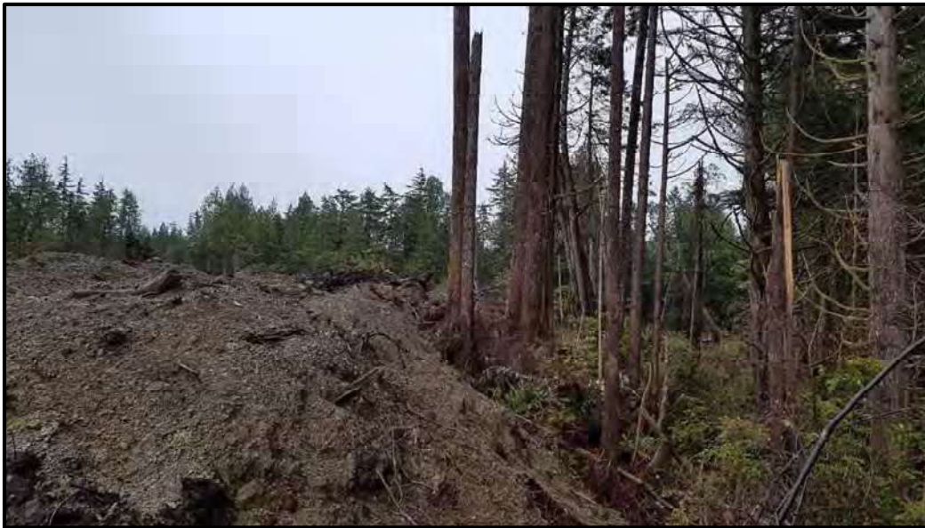
Photo 11: Stockpiled soil burying the base of some trees in 30m foreshore DPA needs to be removed.
