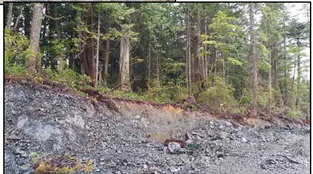
Photo 6: View along main access road; south end of development. Road cleared to edge of 30m highway setback.
